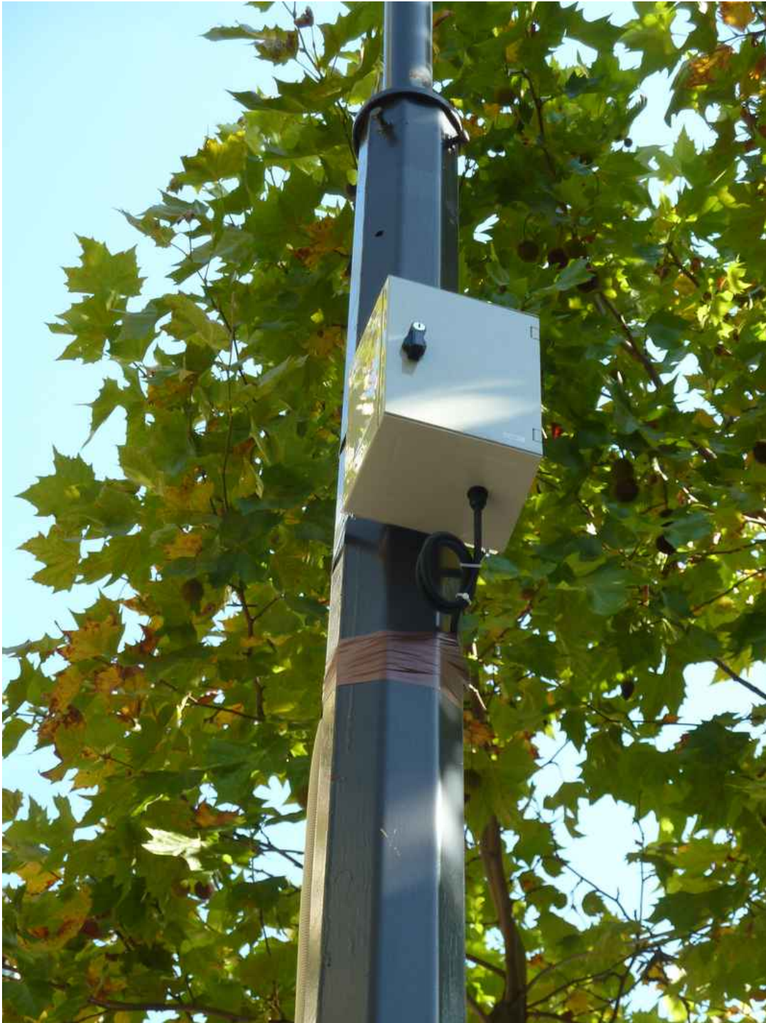
Figure 4.12 – Zoom on beacon B_4 on Friedland Avenue.
