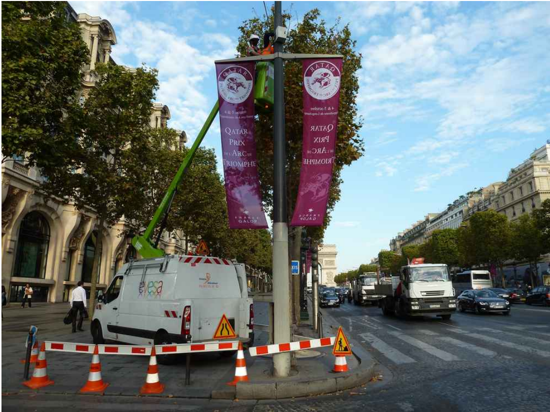
Figure 4.11 – Cradle and workmen installing beacon B_2 on a streetlight pole on the Champs Elysées.
