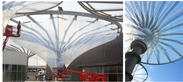
(a) Membrane structure during installation (picture: LEICHT GmbH) (b) Membrane structure after completion (picture: Romain Mesnil)
