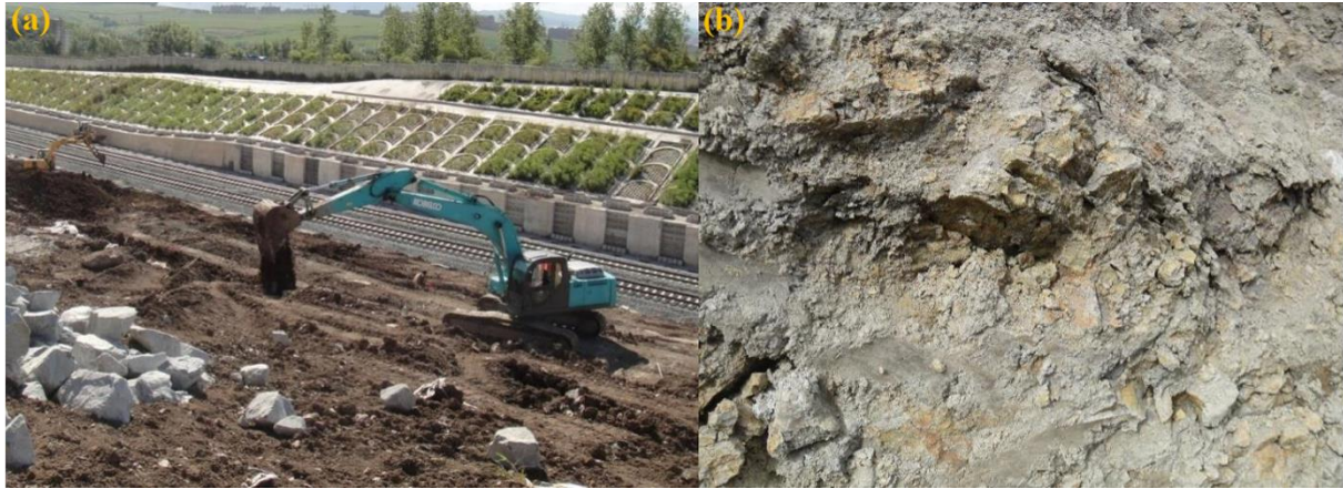
128 129 Fig. 1 Sample site and extracted sample: (a) the mudstone slope at the K275 section of Jilin-Hunchun 130 railway line, and (b) the swelling mudstone in a 4.0 m deep trench 131
