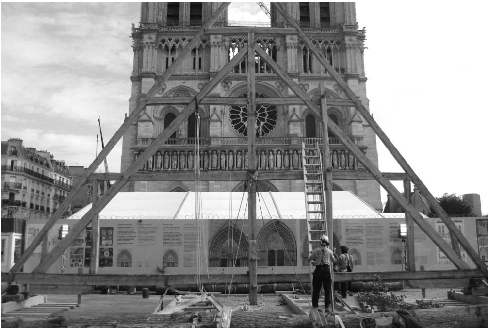
Fig. 10 A copy of N° 7 frame, from Notre-Dame timber frame, built on site on the occasion of French cultural heritage day (September 2020) Photography: S. Caré
