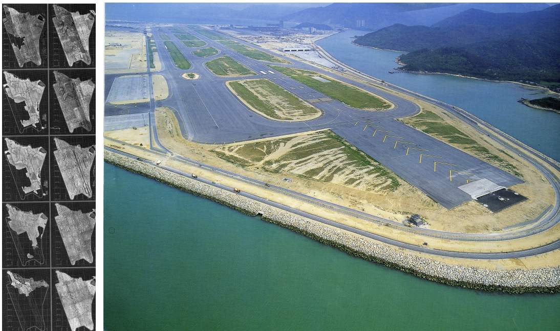
Figure 4. Aerial views and photography of the progression of the airport building site, published in Vision to reality , 1998.
