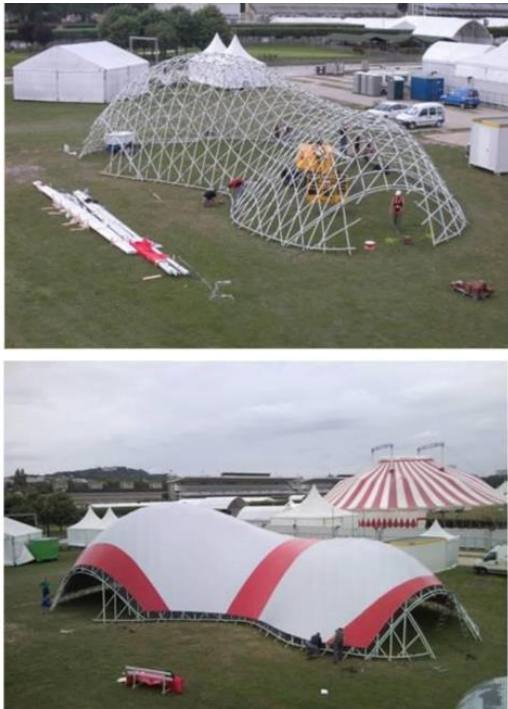
Figure 9. Structural grid achieved and braced (top). Final design of Solidays gridshell (bottom) [23].
