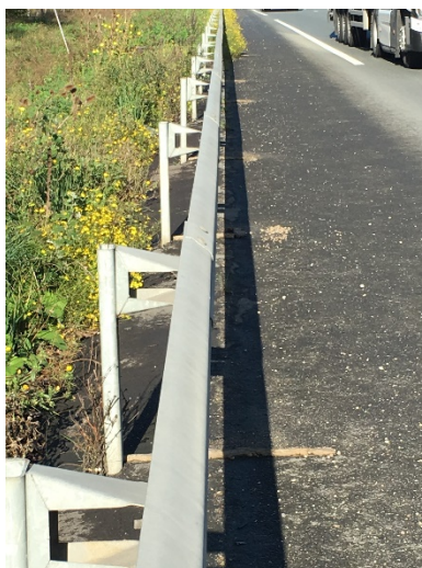
Figure A12. Galvanized steel safety barrier separating the biofiltration swale from the road surface.
