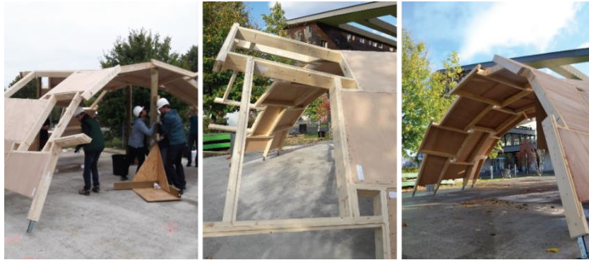
Figure 6. Different stages of construction: tripod with temporary supports (left), cantilevering structure (middle) and completed structure (right)
