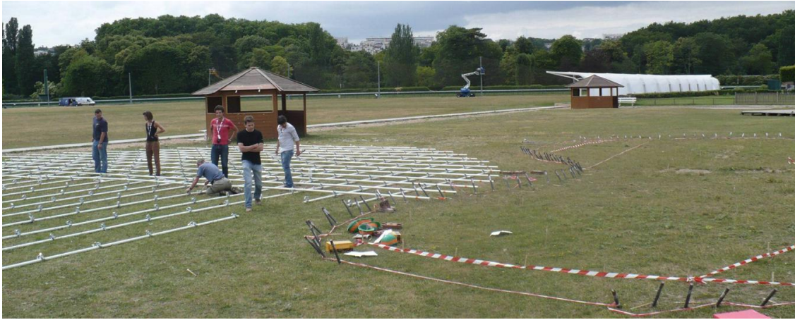
Fig 5. Assembling of the primary flat grid on the ground, near the anchorages
