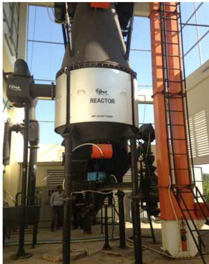
Figure 3: 600kW Gasifier at Golden Daun Keo rice mill, Battambang, Cambodia, 2014-12-20
